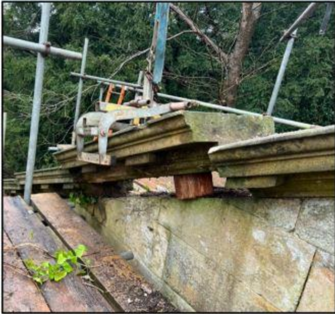
Scaffold not attached to Mausoleum structure.
